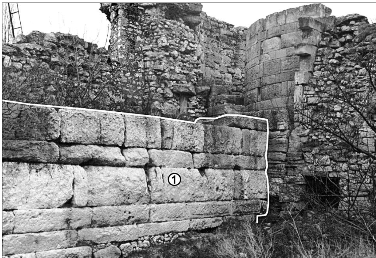
Fig. 5. Curtain 20. View from the interior of the citadel (R. Karasiewicz-Szczypiorski). 1 – remains of the defensive wall constructed in the Roman Period from Inkerman stone.
