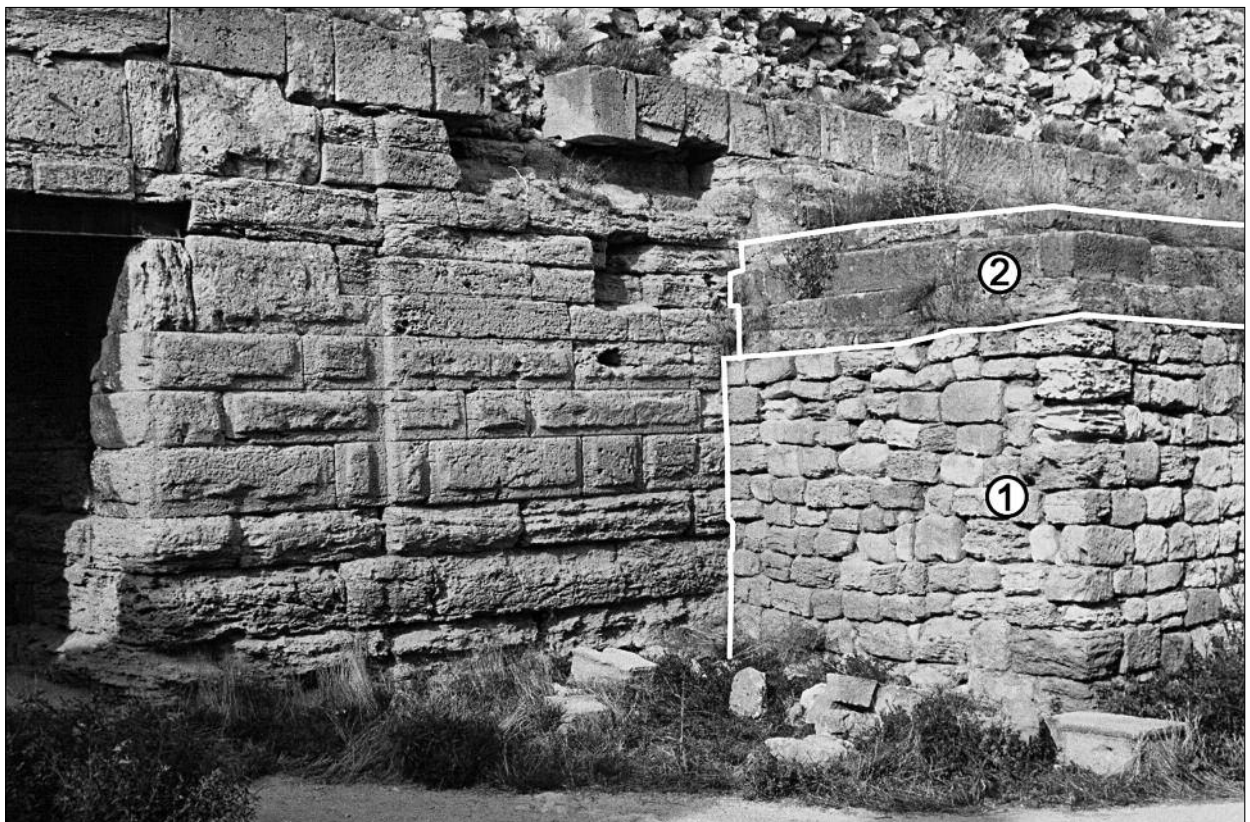
Fig. 4. Curtain 16 and Tomb 1013. View from the outer ward (R. Karasiewicz-Szczypiorski). 1 – walls of the tomb, constructed from roughly cut blocks; 2 – upper part of the structure, made from regular blocks.
